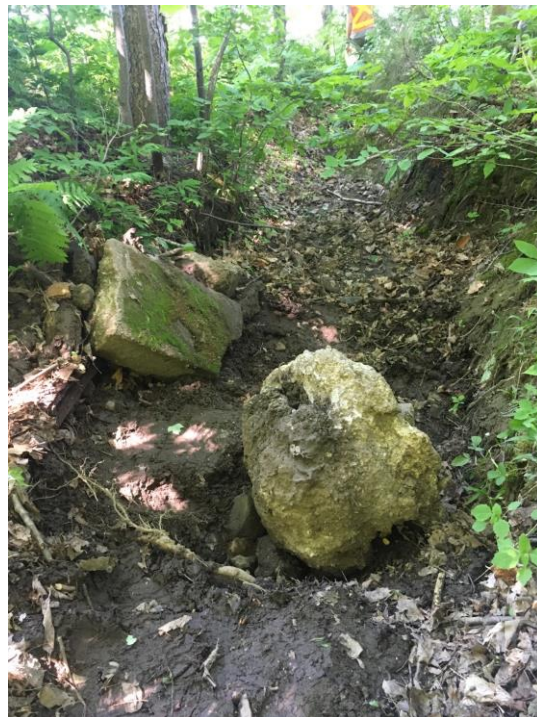
Figure 8: Erosion in the swale downstream of Camp Road. The concept design for this area (SW-5) describes BMPs that would stabilize erosion and treat runoff.
